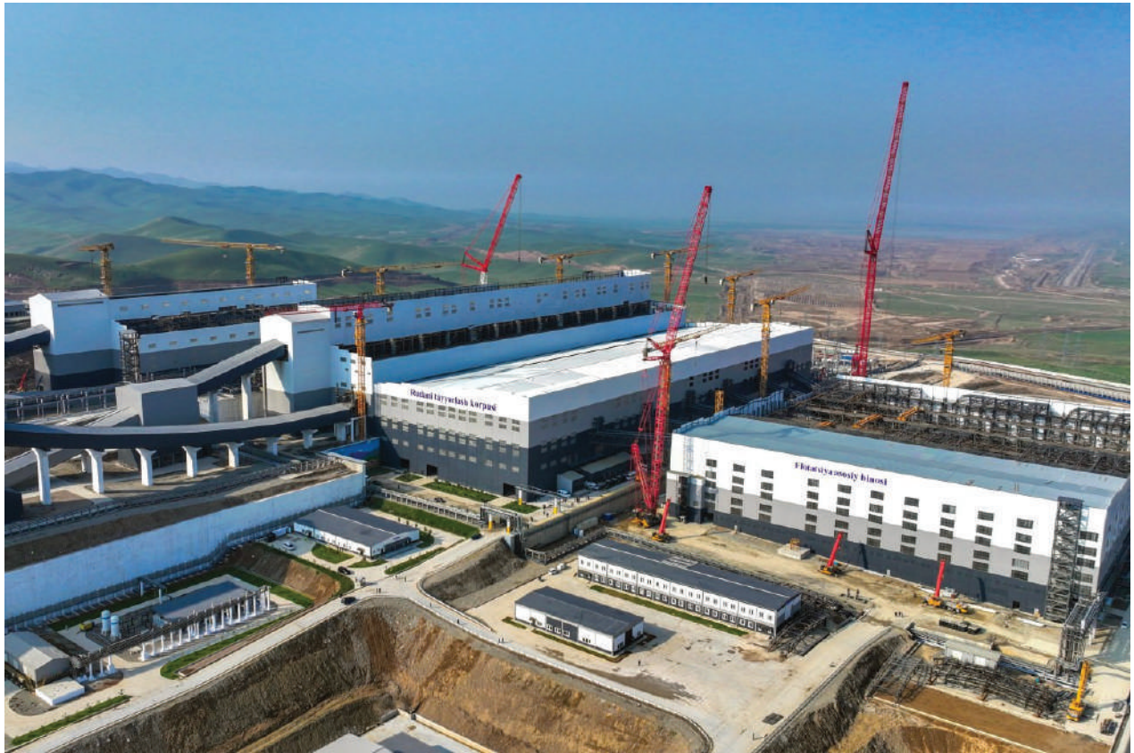
Copper Processing Plant No. 3 at the Almalyk Mining and Metallurgical Complex in Uzbekistan. Source: president.uz
