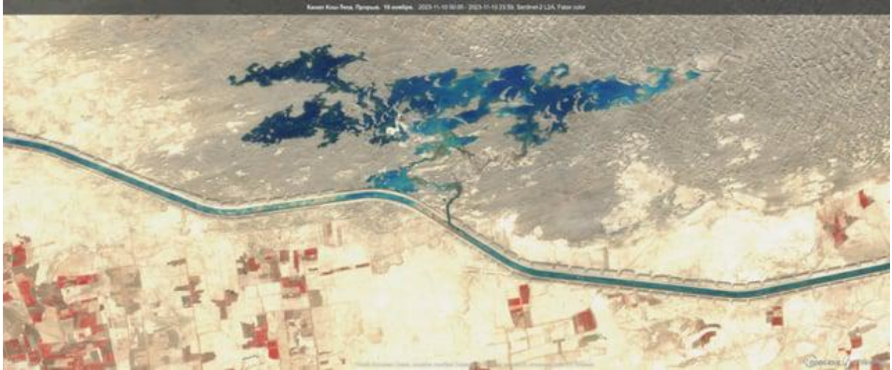
The $684 million canal breached its walls, creating a massive lake in October 2023. (Copernicus Sentinel satellite photo)
