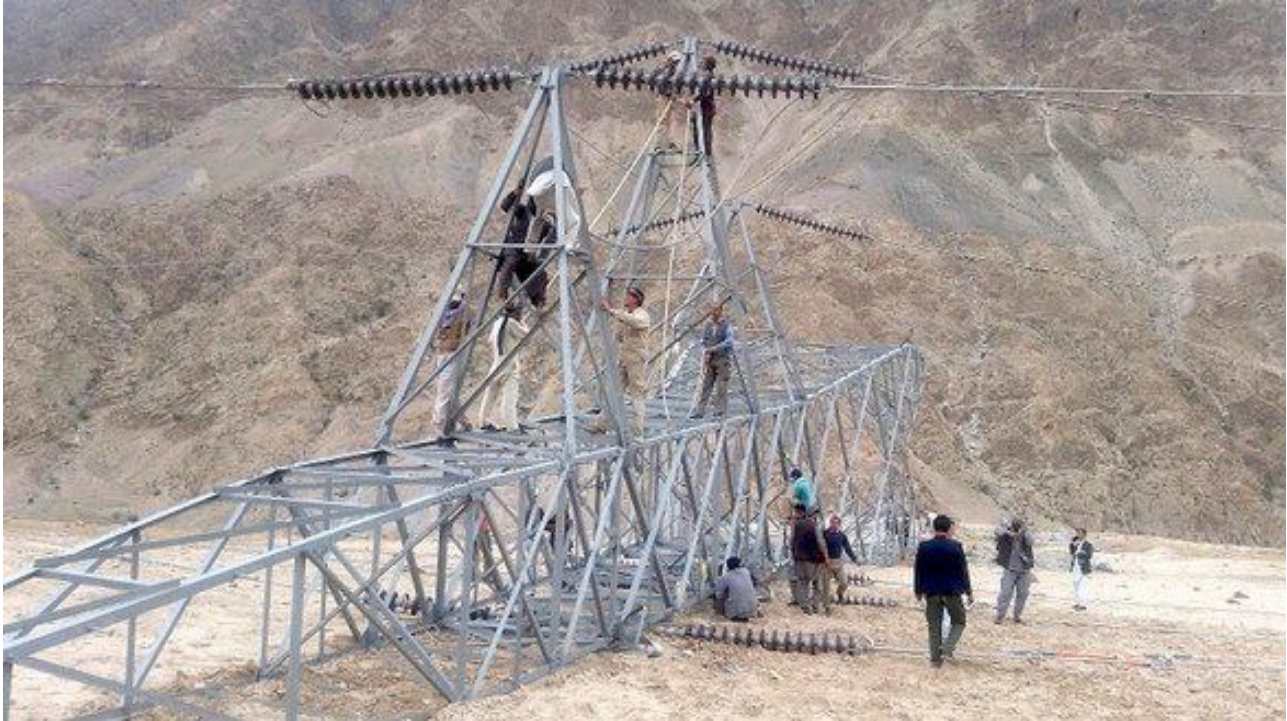
A Da Afghanistan Breshna Sherkat (DABS) technical team was able to temporarily reconnect power lines on April 15 in Baghlan Province. Work is under way to permanently resolve the problem, said DABS. [Source: DABS/Facebook]
